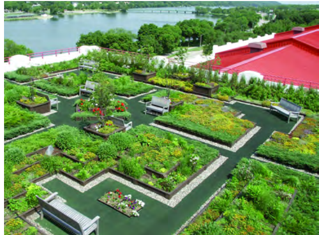
Fig A.6.c.1 and 2: A modular vegetated roof system reduces stormwater and insulates the roof surface.
