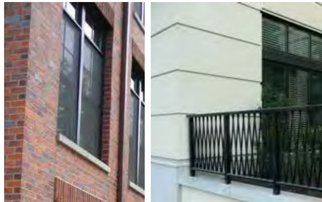
Fig. B.5.c.2. Façades exhibiting long-lasting timeless materials such as brick and stucco.
