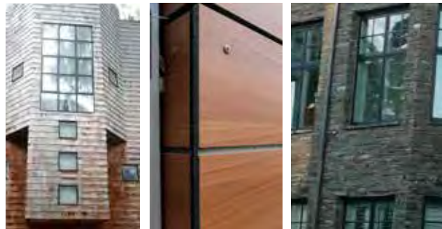
Fig. B.5.c.1. Façades exhibiting long-lasting materials such as wood siding, wood veneer, wood shingles, and stone.
