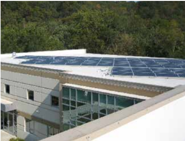
Fig. C.1.D.2: A roof using solar energy panels on a "white roof" to minimize heat gain and reduce cooling costs.
